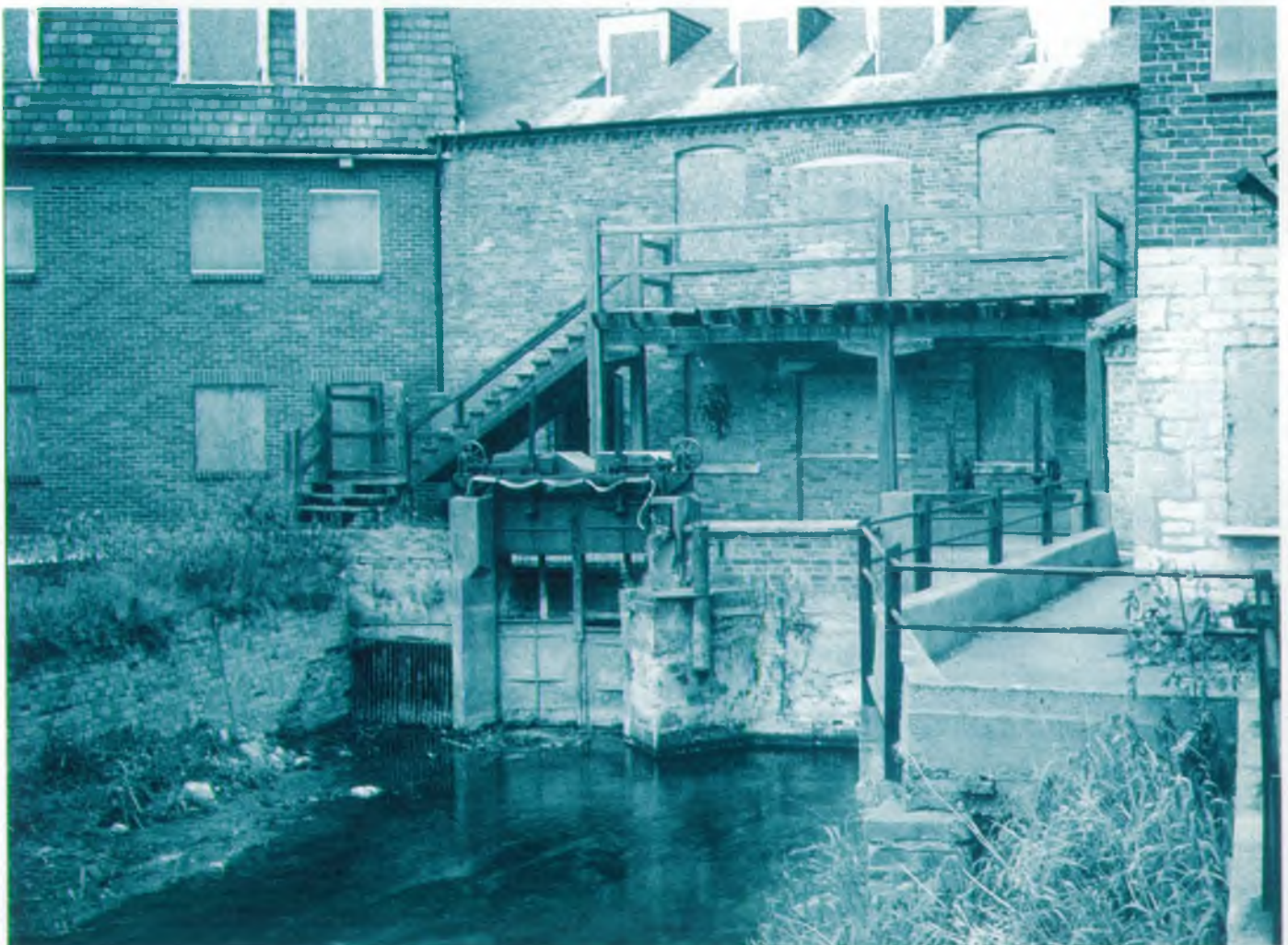
Navigation structure impeding fish pass
