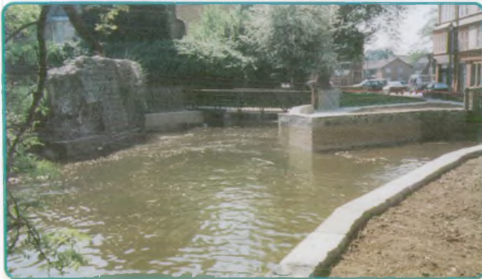
◁ The final result with the old Abbey wall in the left of the picture
