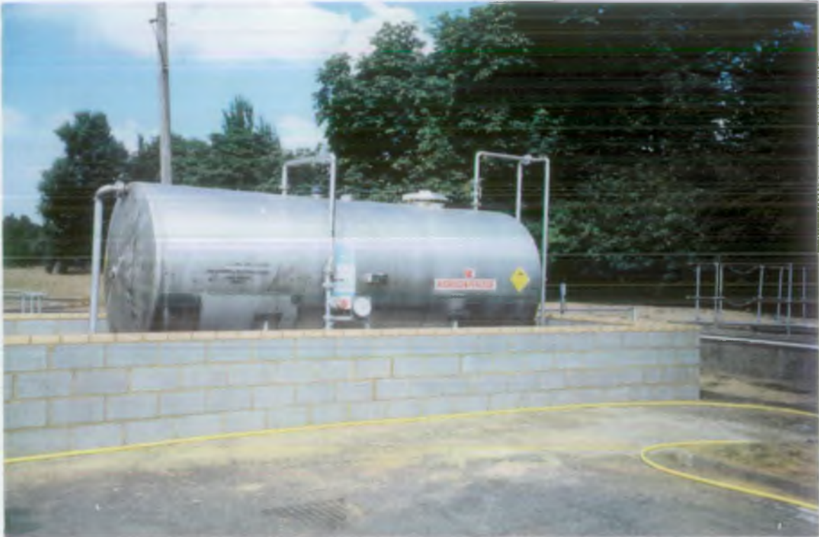
Plate 3: Hydrogen peroxide dosing facility at Kew STW
