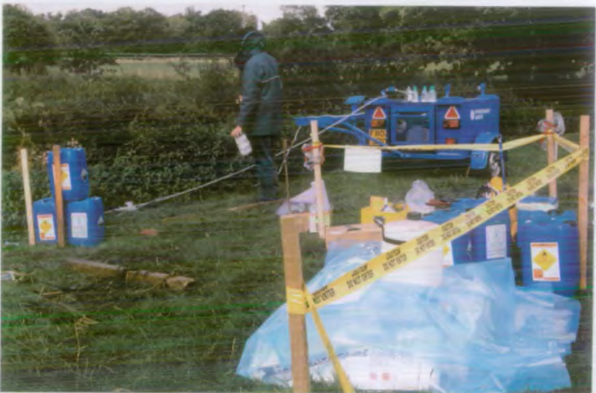
Plate 8: Hydrogen peroxide storage area
