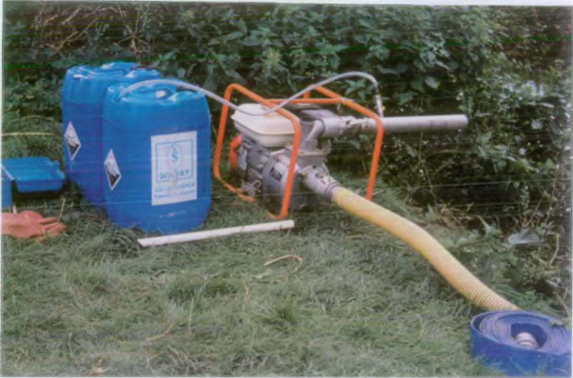
Plate 7: Venturi based hydrogen peroxide dosing system
