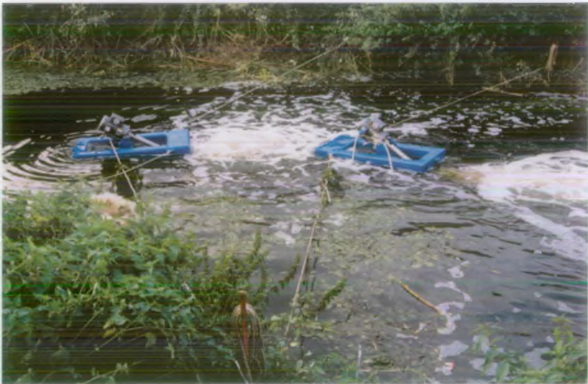
Plate 4: Tornado turbo-aerators in the River Mole at Kinnersley Manor
