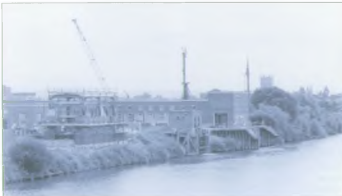
Mythe Water Treatment Works at Tewkesbury
