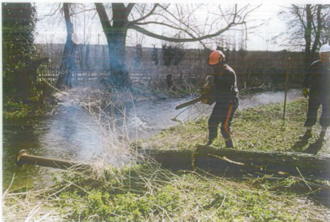
Picture 9 Tree Pollarding on the River Darent at Horton Kirby. Use of chain saw in immediate vicinity of river.
