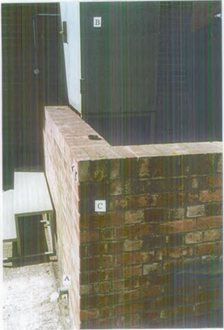
Picture 3 Leigh Office bulk oil tank bund. A - rain water drain through bund wall; B - fuel dispensing cabinet; C - bund wall.
