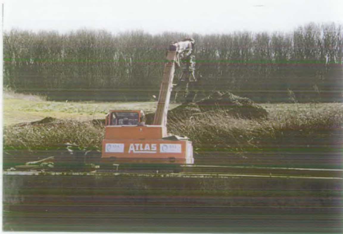
Picture 10 Dredging from "Bourne 2" on the midway below Oak Weir. Spoil is deposited on the river bank.
