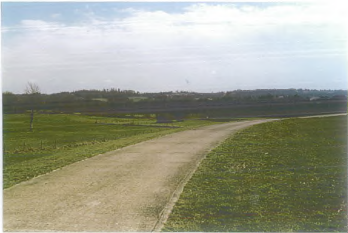
Picture 1 Leigh Barrier earth embankment south of main river course, showing starkness of structure.
