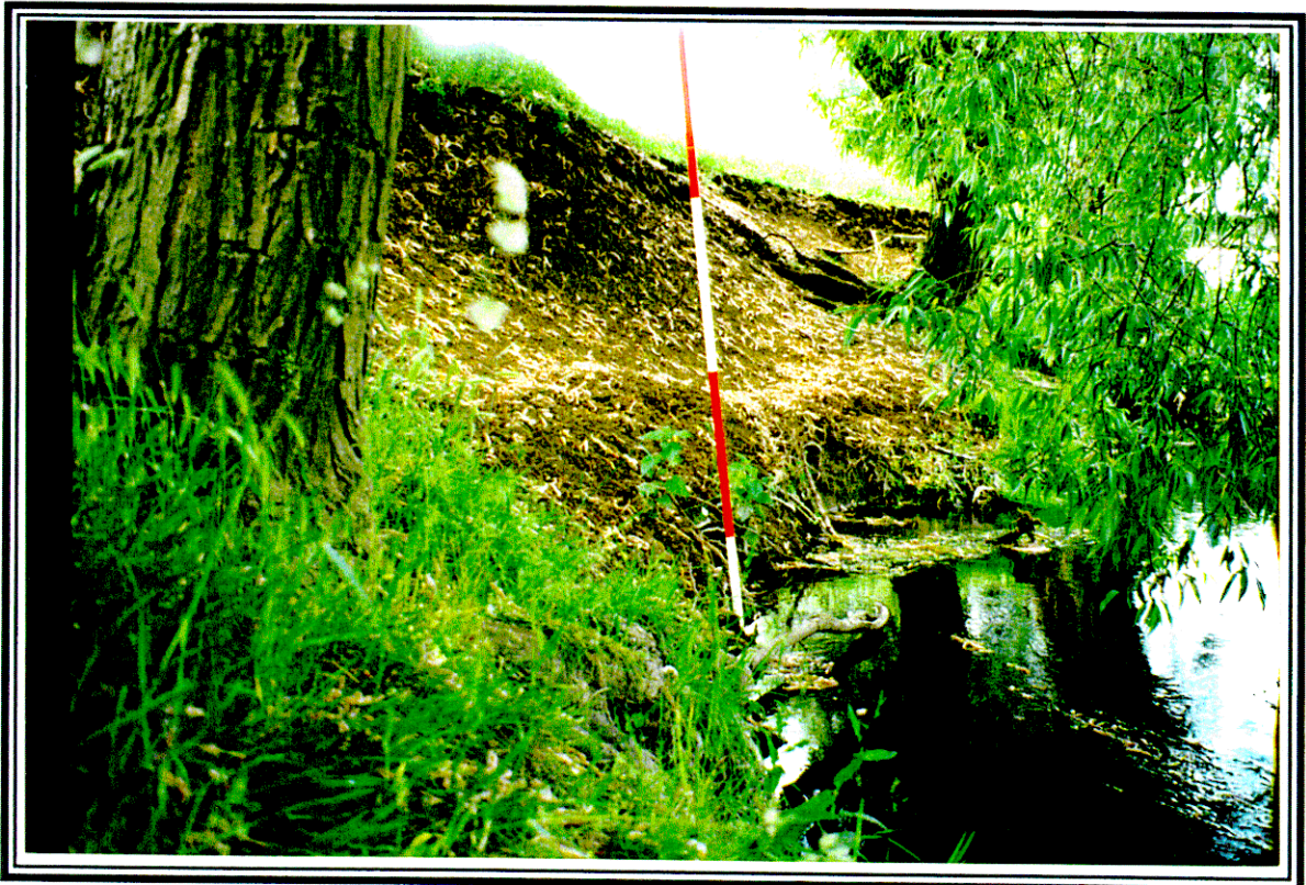
Plate 2: River Ouzel (Milton Keynes Valley Park) - corrosion (and not rotational slide) appears to be the process. Note the exposed lateral roots of the distant willow and the mature, rigid bifurcating roots of the nearside willow
