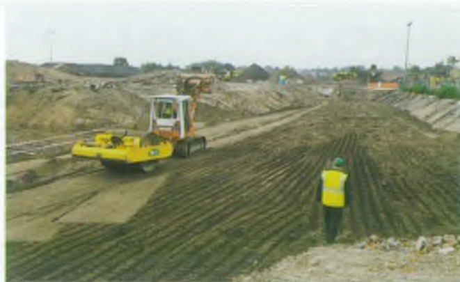
Above Basford gas works site, Nottingham - Replacing washed soil from the soil washing plant, after remixing coarse and fine components
