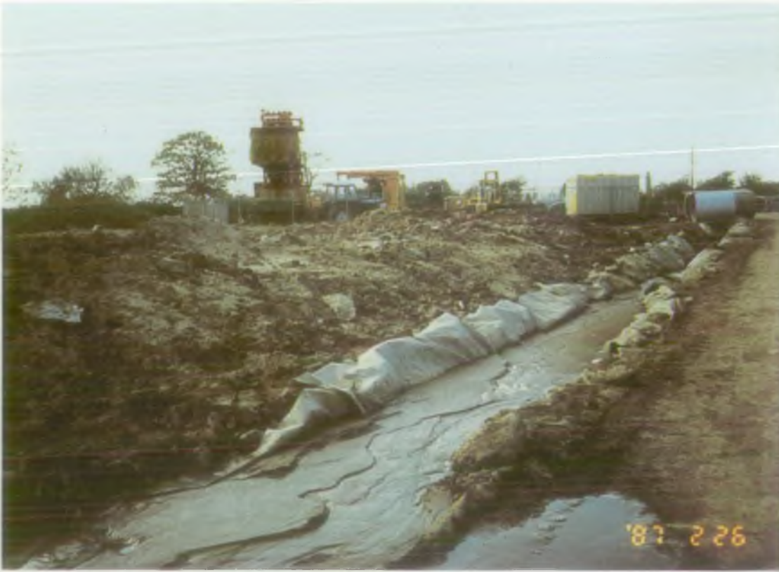
Silt from motorway construction. North West Region
