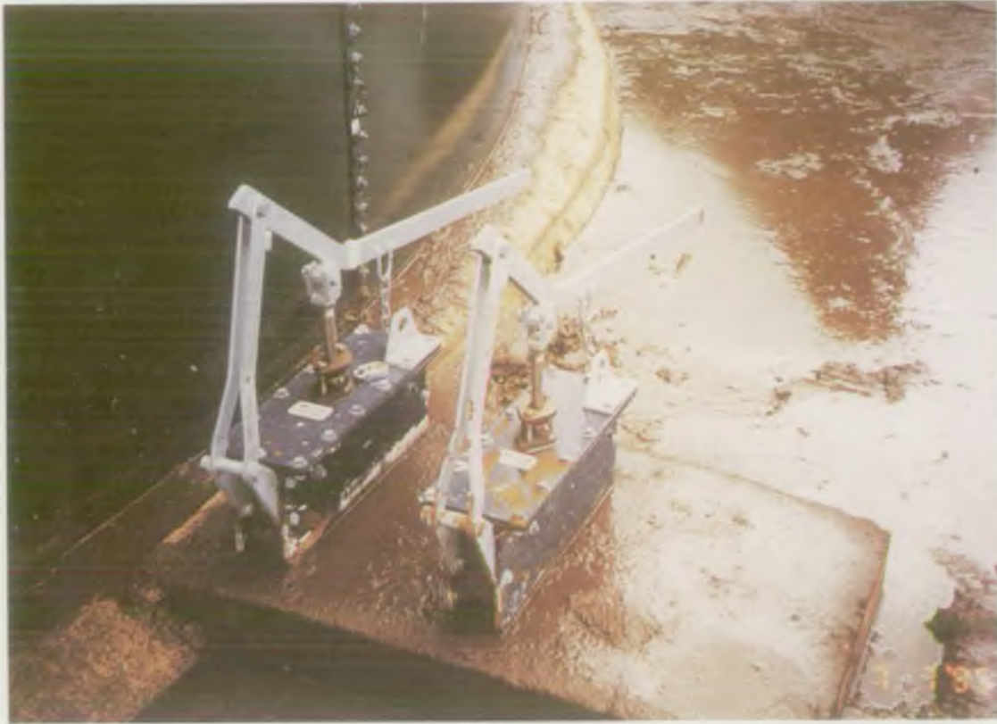
Plate 5 Aberystwyth farm incident – vandalised valves
