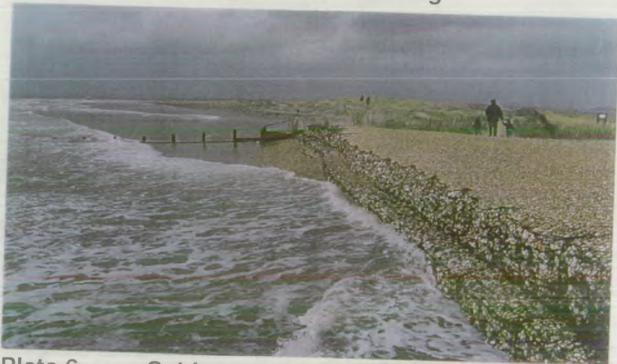
Plate 6 Gabions at the neck of East Head
