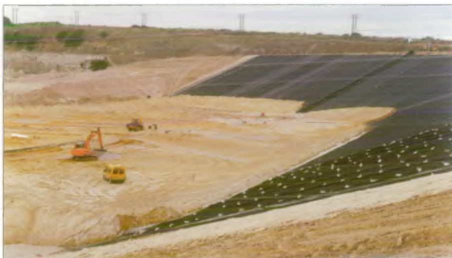
The lining of a new landfill on the Chalk with an artificial membrane in order to protect groundwater.
