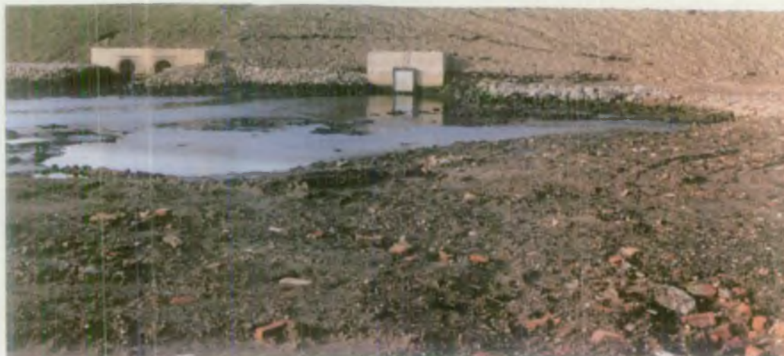
SOUTH EAST CELL SLUICES, LANDWARD SIDE - MARCH '95 ORIGINAL TWIN REPLACEMENT ON LEFT ADDITIONAL SLUICE ON RIGHT
