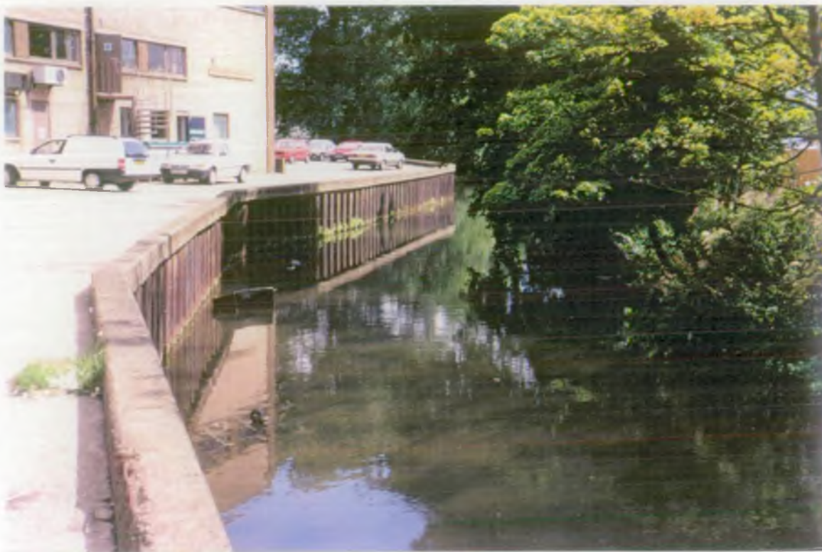
PHOTO 11 - Industrial trolley and bin in river. Grid Ref. (0604,0537).
