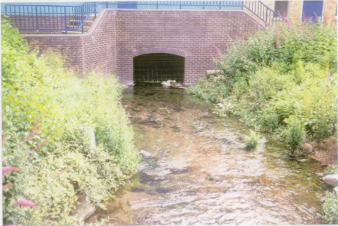
PHOTO 3 - Small quantity of foam visible from road bridge. Grid Ref. (8429,9399).
