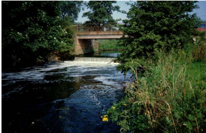
Figure C1 - The invert of the box culvert acting as a weir
