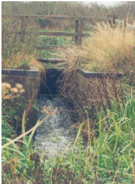
Figure A6 - The fish pass looking upstream towards the canal
