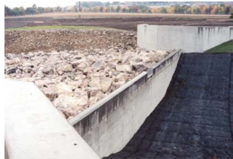
Figure F2 – View of recently constructed weir showing concrete structure and rock downstream
