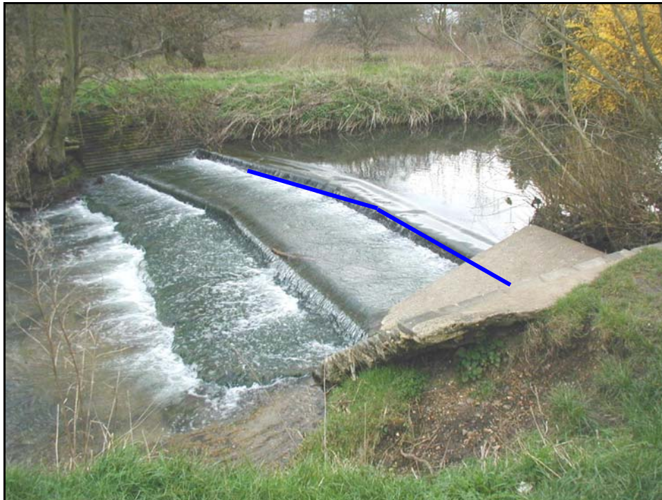
Figure P2 – Undermining at rigid revetment and lack of scour protection downstream
