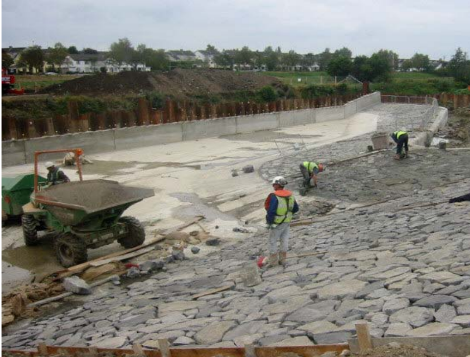
Figure K2 – Similar to Figure K1 at a later stage of construction, with masonry facing in place
