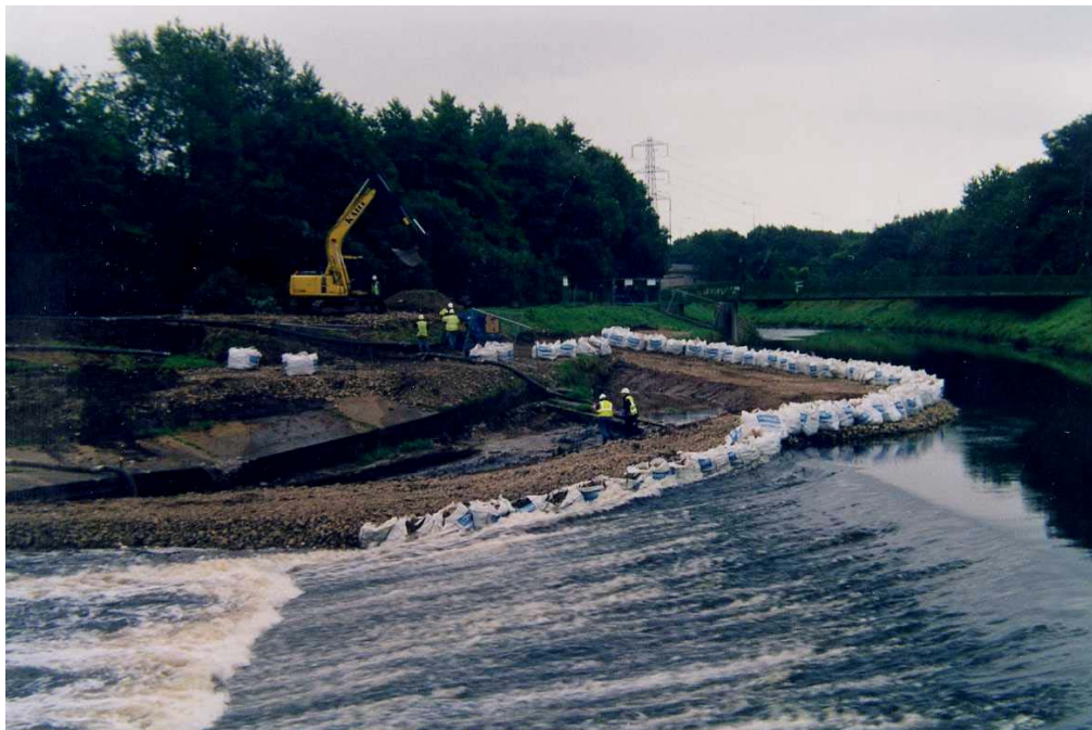
Figure L1 – Part of the weir isolated by a cofferdam to allow remedial works to the weir and the construction of the fish pass
