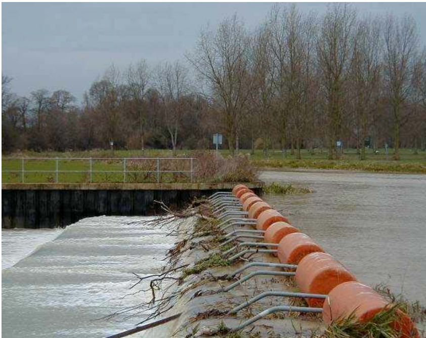
Figure 2.2 Safety boom upstream of a weir
