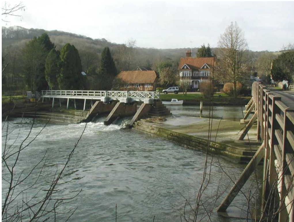
Figure 2.22 A large gated weir on the River Thames
