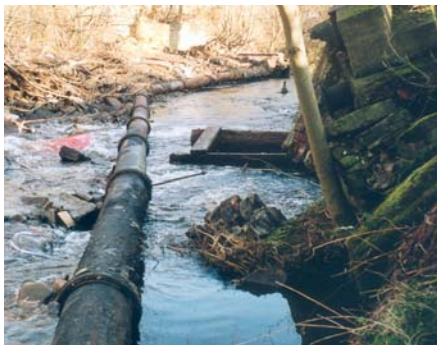
Figure E2 - View from upstream of weir, after breach.
