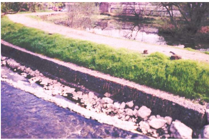
Figure E6 - State of weir, April 2002
