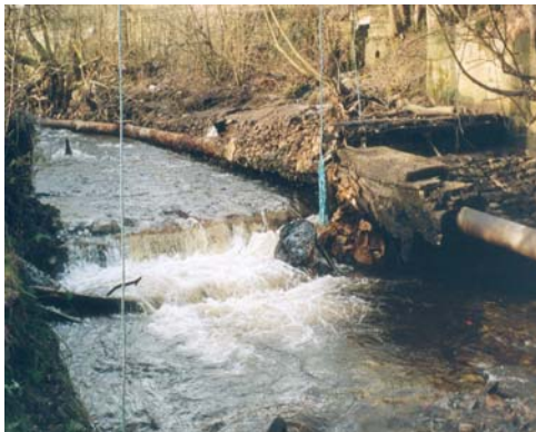
Figure E1 - Weir breach viewed from downstream.
