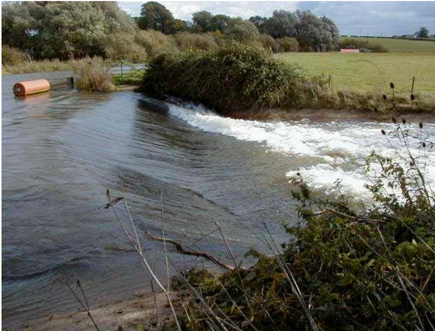
Figure AD5 - Side weir in operation
