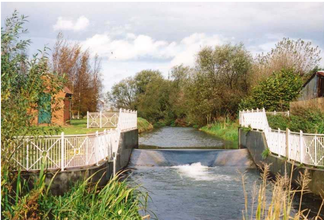
Figure 1.3 Gauging weir at Horncastle
