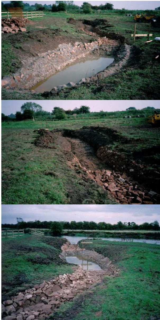
Figure A4 – Three photographs of the construction of the bypass channel and pools
