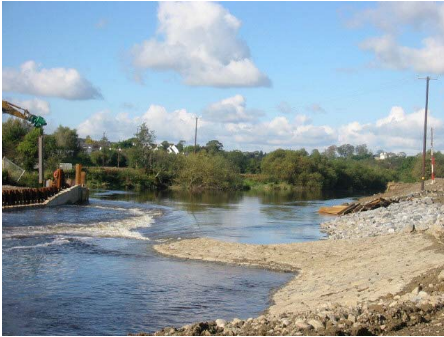
Figure K4 – Flow diverted over the completed left-hand side of the weir
