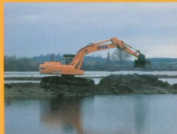
Overburden being re-profiled to provide a platform for the reedbed, Source: English Nature
