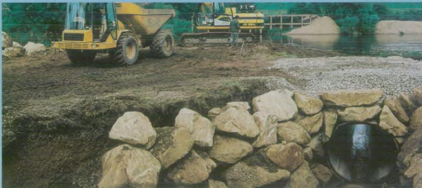
The pipe links Marina Pond, Holme Pierrepont to the River Trent
