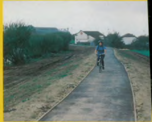
A hard surface has been laid on top of the flood defences which begins at the Trent Port Pub
